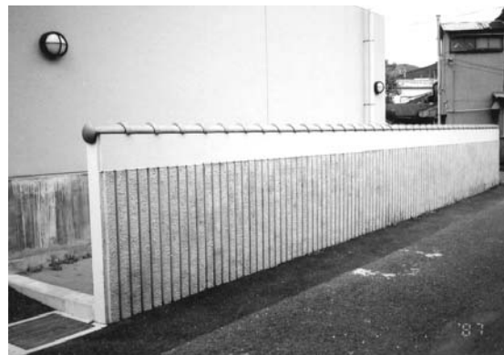
Photo 13. Fake stone wall made of concrete
